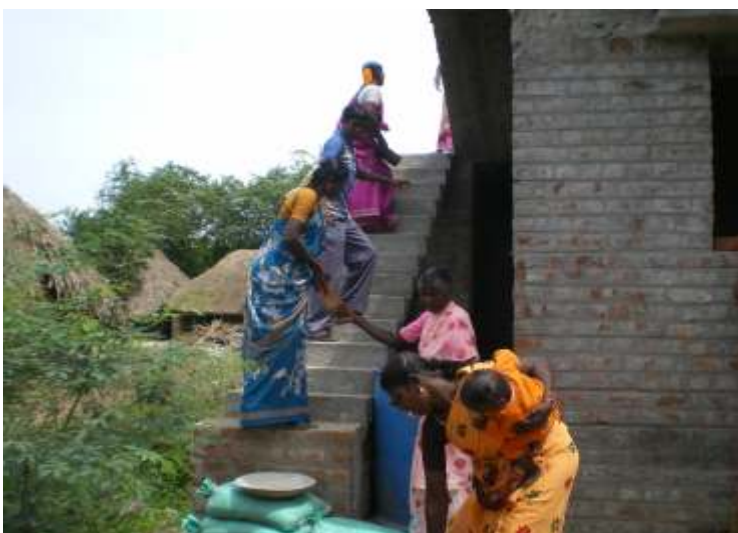
▲ 70 homeowners along with REAL Staff (NGO partner) join hands to participate in the Home Partner's Build at Periyathachur village
