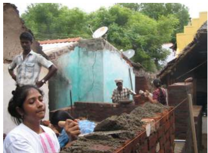
▲ College students volunteer for a day to participate in the Students Build on 20th September'08 in Kammappatti, Chennai.
